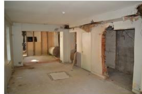
03 Unauthorised works. View inside Room 11 of Woodcote Cottage of the crudely extended opening to the original stable block.
