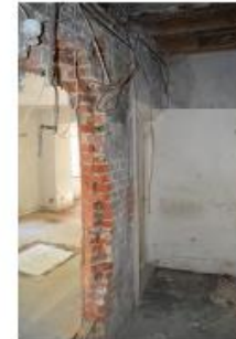
04 Unauthorised works. View inside Room 14 of the original stable block opening, widened.
