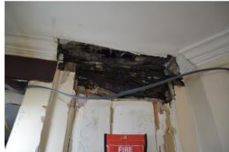
01 Opening up works. Rotting timbers in Room 2 ground floor of Woodcote Cottage caused by water ingress at second floor roof level.
