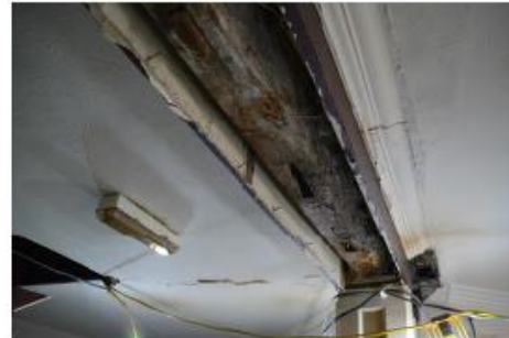
02 Opening up works. Timber casing to beam between Rooms 2 and 4 of Woodcote Cottage showing mortise evidence of a former wall.
